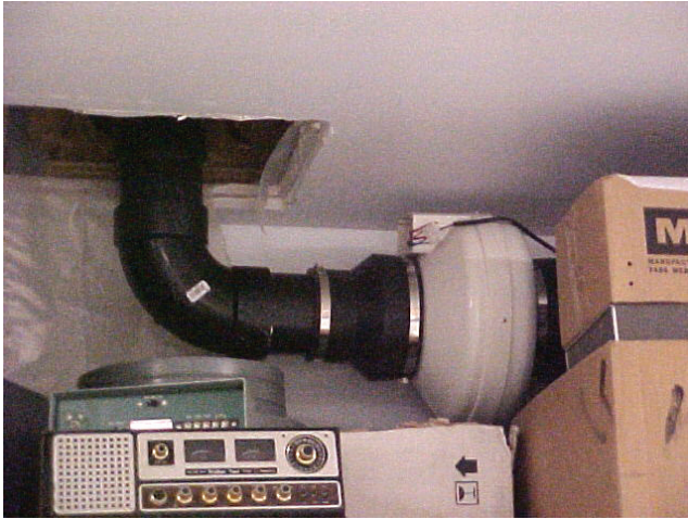
Figure 7. A photo of the axial fan and exhaust piping that removes radon from Dale Powell's sub-slab area as a result of his radon mitigation effort. The pipe ultimately dumps the radon-laden air outside.
