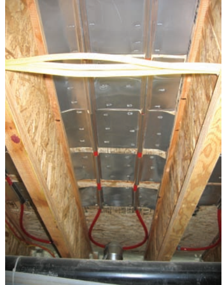
Figure 4. A view of the heating distribution system, viewed from under the first floor. A loop of polyethylene PEX® pipe is backed by an aluminum heat transfer surface/plate, which is stapled to the underside of the wood floor. The aluminum plate aids in heat transfer.
