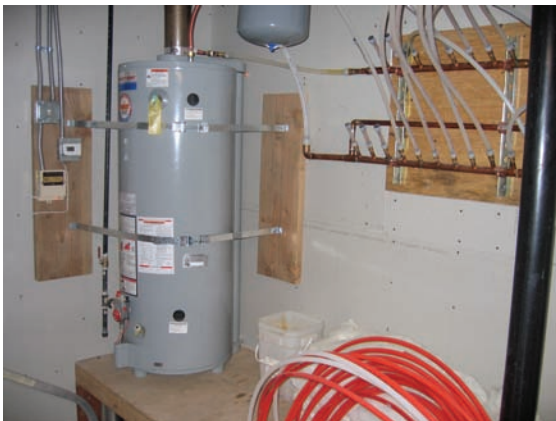
Figure 3. The water heater (using propane) heats the house using an in-floor heating system. There is no boiler or furnace.
