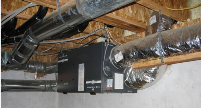
Figure 2. The heat recovery ventilation (HRV) system in the Homer house.
